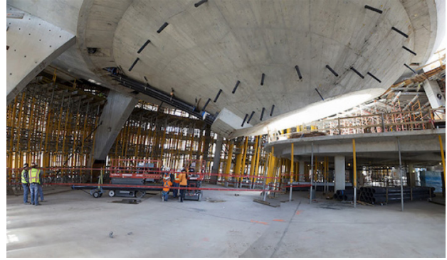
Figure 27: Philip Frost Museum of Science, Florida, Digitally Fabricated Formwork & Cast-In Place Concrete Construction
